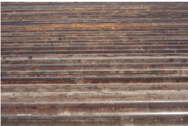
Figures 1 & 2: Examples of red rust on pipe
