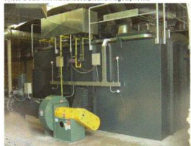
RTO scrubber system.
